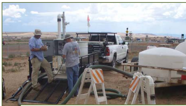
EPA Region 9 investigation of LUST-contaminated soil and groundwater affecting Navajo Nation and Hopi Tribe tribal lands near Tuba City, AZ, involved use of a conceptual site model and mobile laboratory to guide subsurface application of food-grade vegetable oil that accelerated bioremediation of contaminated soil.
