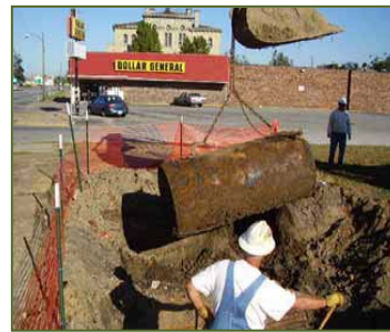
Surgical excavation and tank removal at the G&L Clothing site in Illinois allowed for minimal site disturbance and maximum recycling or reuse of excavated materials.
